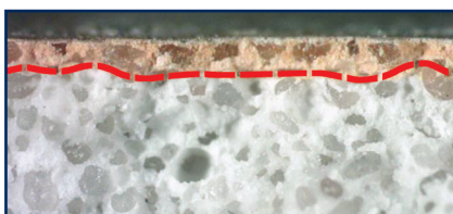
Petrography of freshly fractured cross-section of FloorEverDri treated slab. Beige-colored paste at the surface (above red line) repels water due to FloorEverDri penetration, while off-white paste not affected by the sealer (below red line) exhibits high water absorbency. Courtesy CTL Labs
